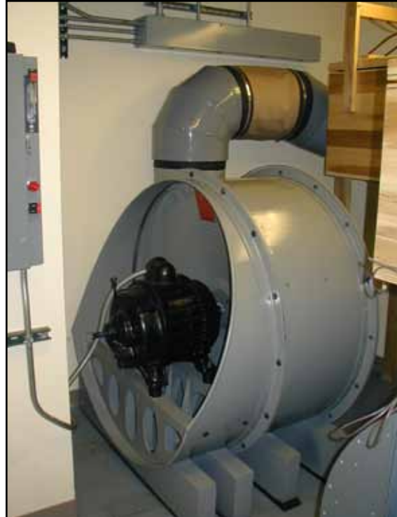
newly-installed Spencer blower for Orchestra Hall, Chicago
