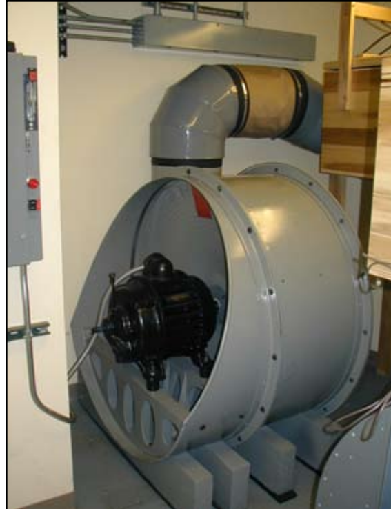
newly-installed Spencer blower for Orchestra Hall, Chicago
